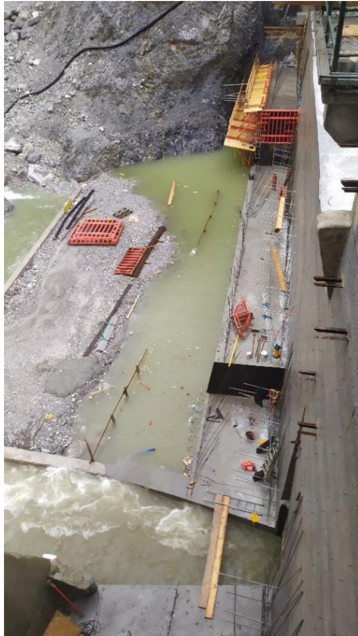
Figure 8 – Flood in the upstream dam site (with the firsts dam segments)
