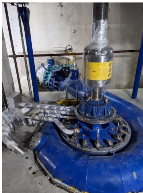
Figure 2 – Francis turbine – Cugno-Brembo Concession
