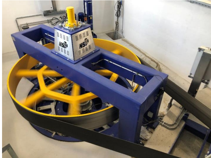
Figure 5 – Belt transmission at Urago plant
